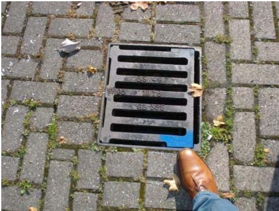
Picture: Colour-Coded Drain Covers
