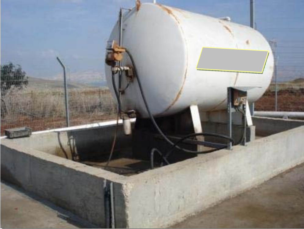
Picture: Effective Containment of a Tank
