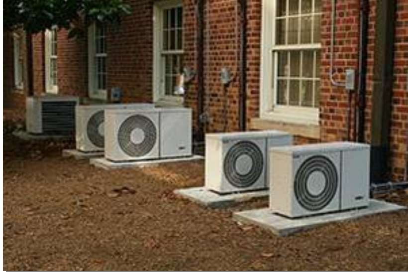
Picture: Example of ODS-Containing Equipment
